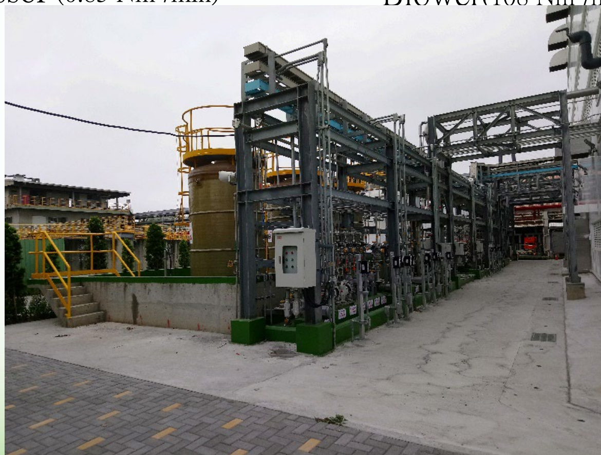
Chemical Tank & dosing pump area
