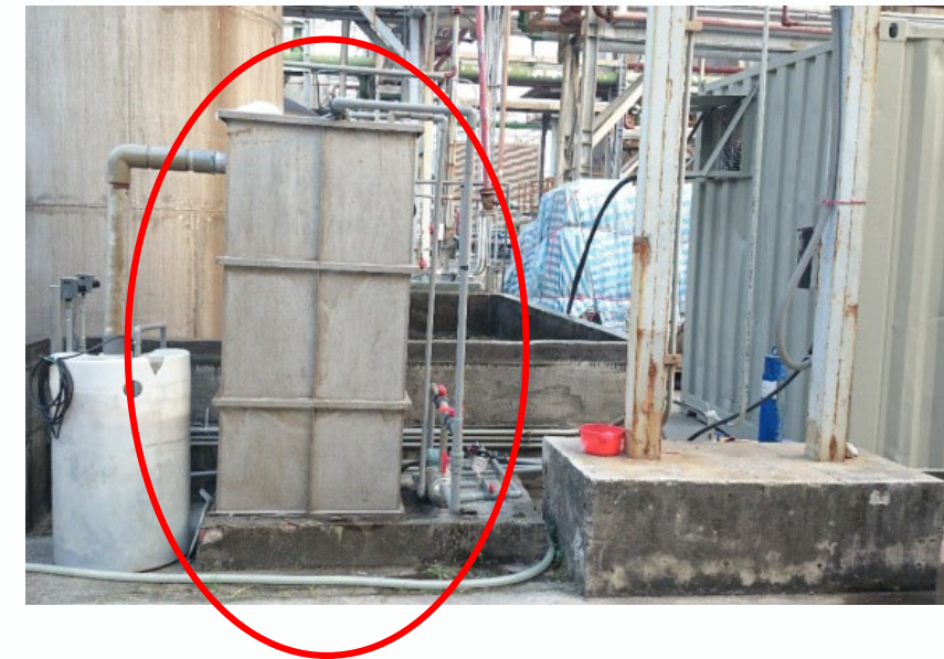
Submerged membrane Filtration Tank
