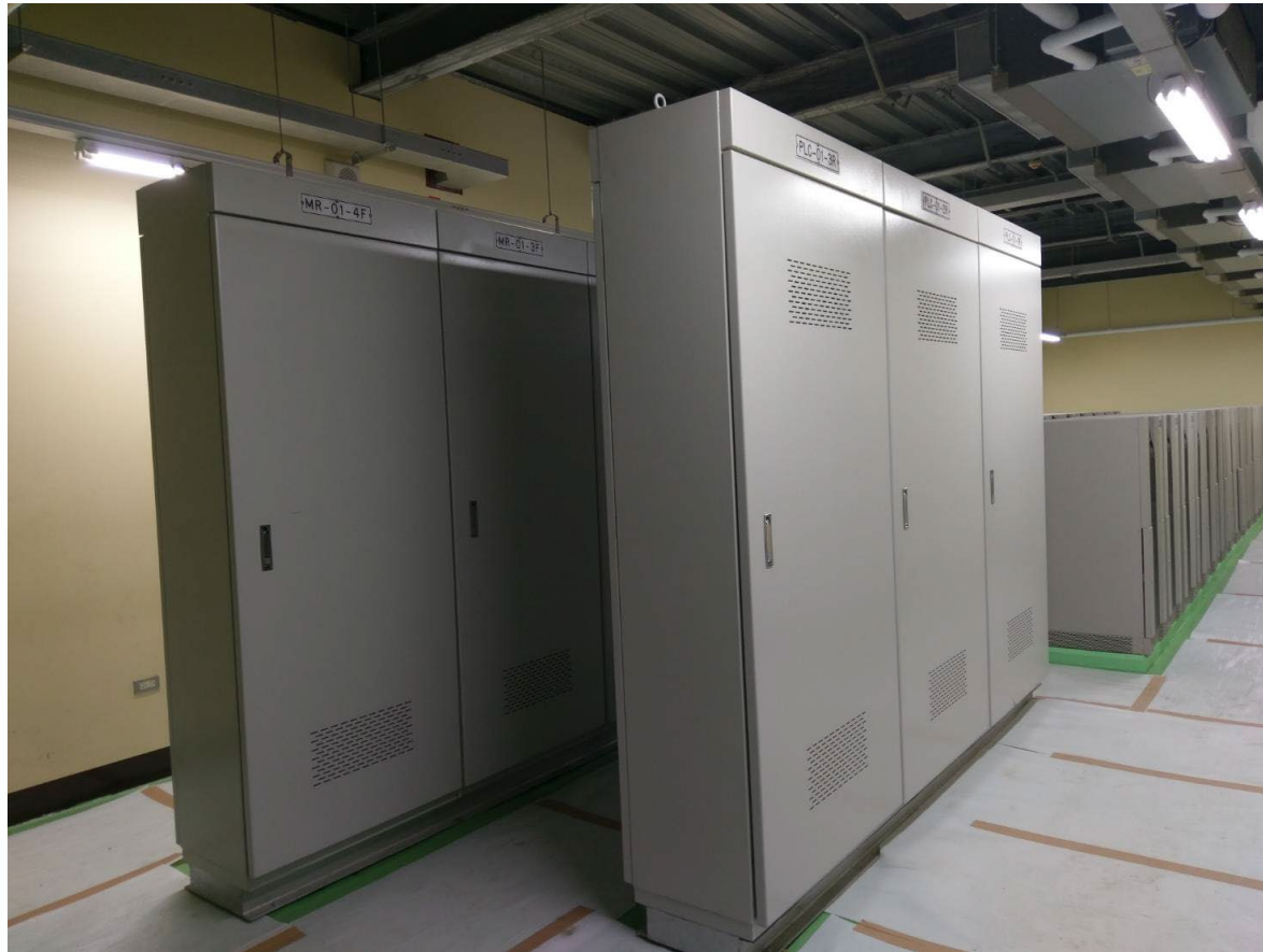
PLC panel and Marshalling cabinet
