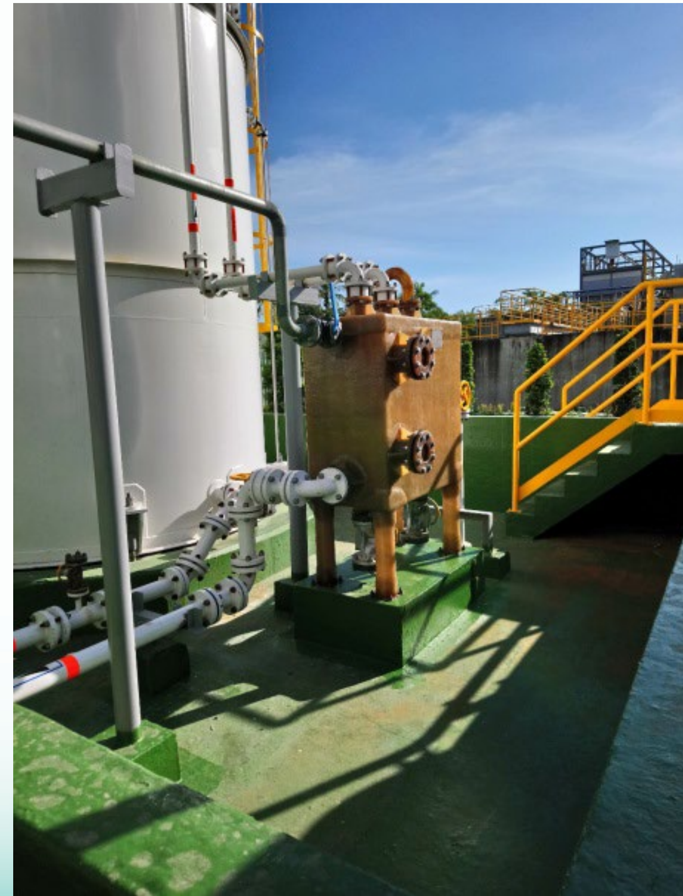
HCl Tank & water seal tank
