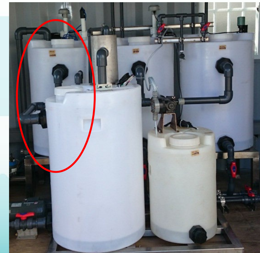
EDR Influent Tank
