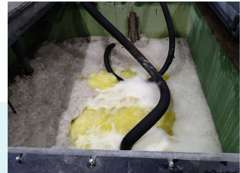
Cleaning with 1% citric acid for 1 hour in SMF immersing Tank (TK-9302)
