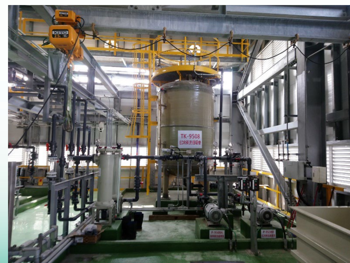
EDR CIP Tank
